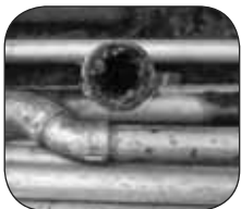
Corroded steel pipe
